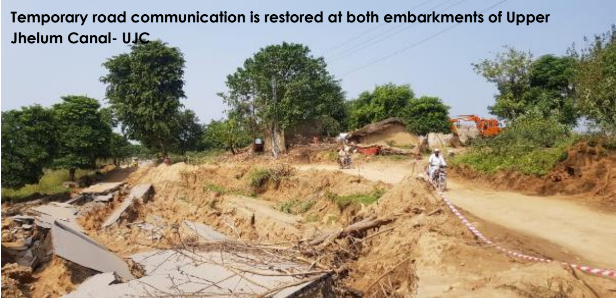
Machine is stuck due to soft soil and rains during the rehabilitation work of UJC embarkments'
